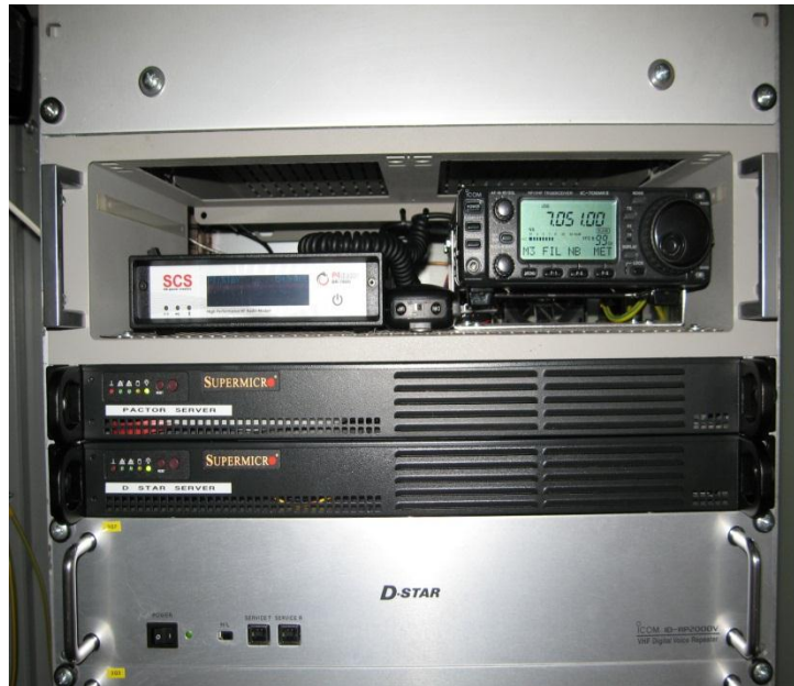
Pactor Anlage HB9AW
